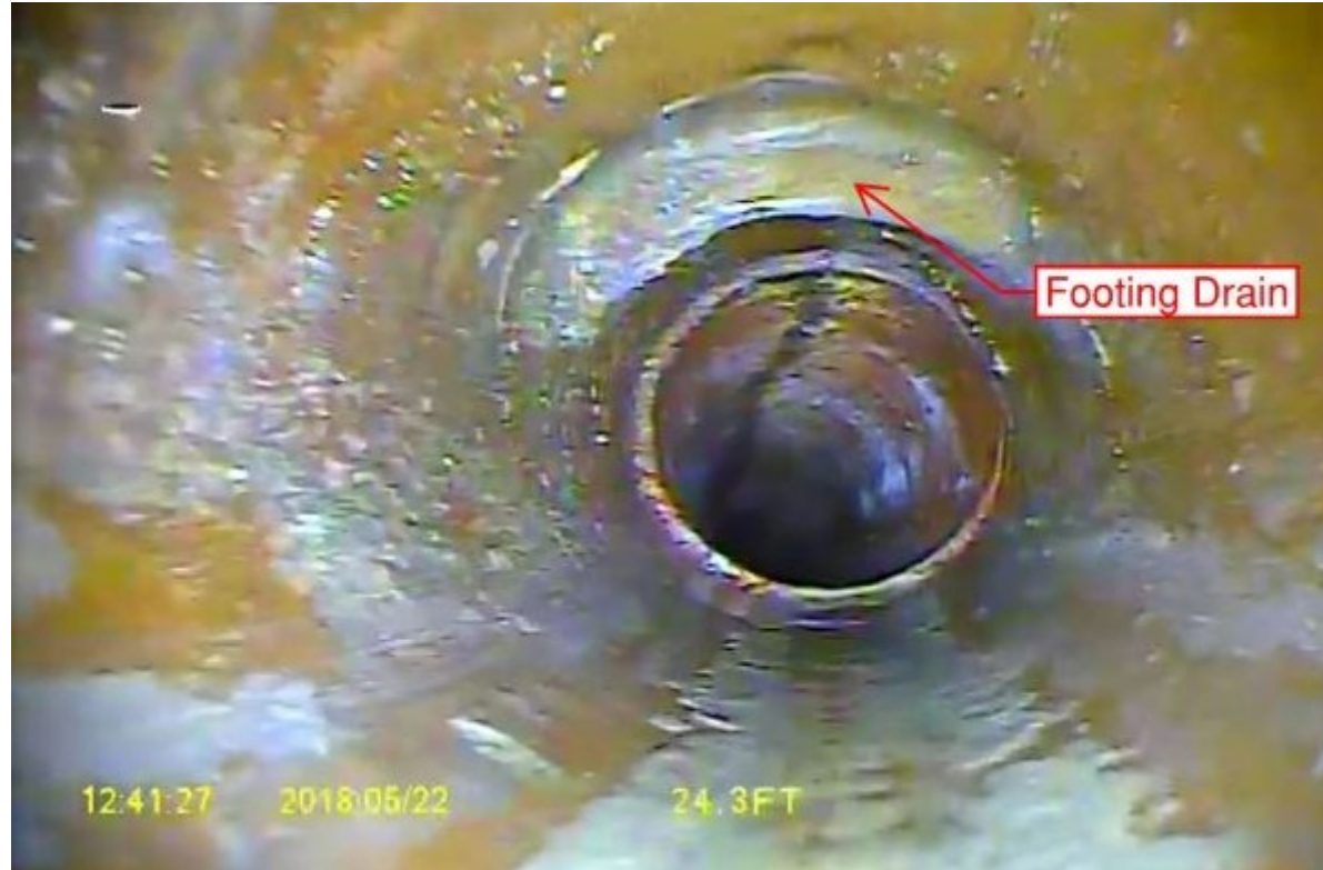
Tap in Lateral Past Foundation IMPROPER
